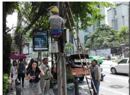
Aerial Optical Fiber Cable
